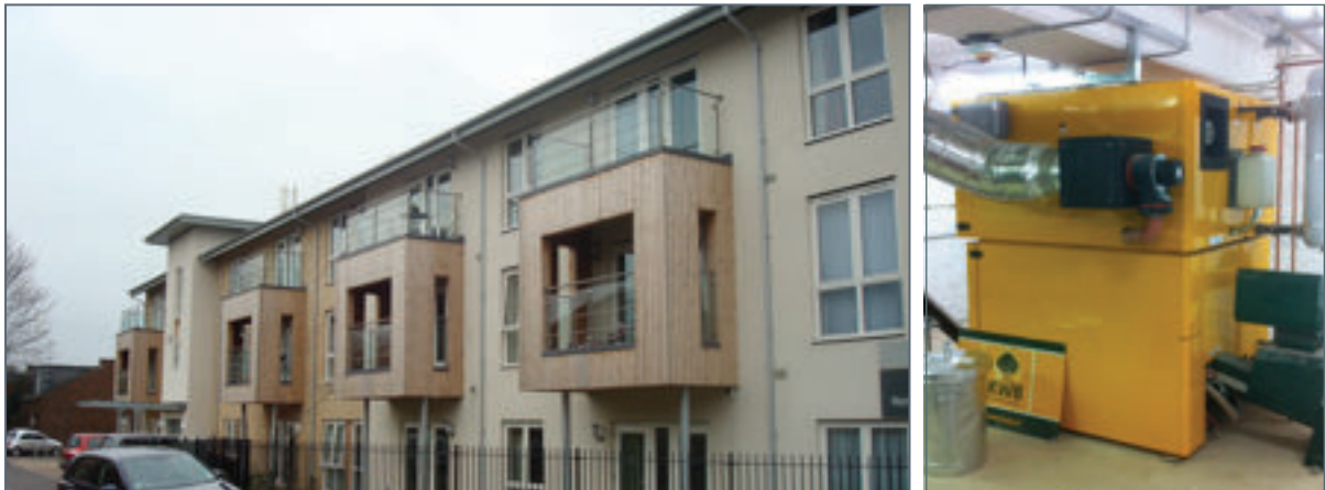
Photo 1: Front elevation and biomass boiler, Richard Newcombe Court, Cambridge.
